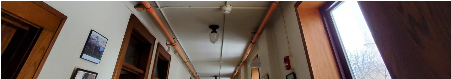
Residential retrofit in the fire station using CPVC pipe protects sleeping firefighters.
