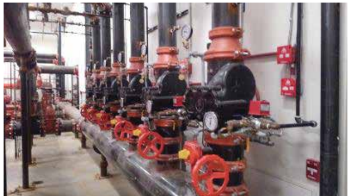
Foam-water deluge systems protecting the entire hangar floor space. Each deluge system protected an area over 9,000 square feet each.
