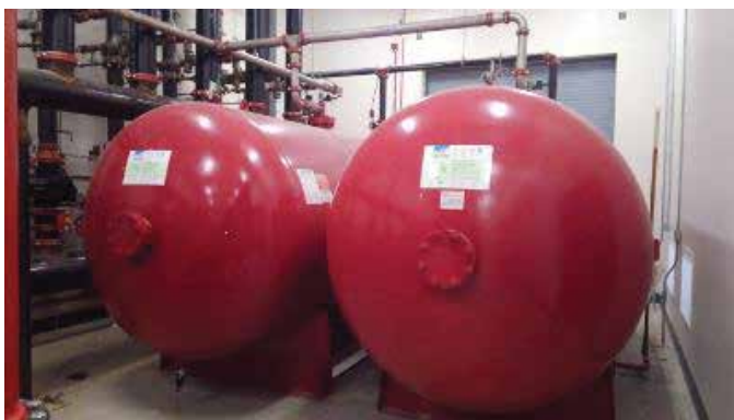
Two 2,600-gallon bladder tanks containing a total of 5,200 gallons of RE-HEALING 3% Fluorine-free foam.
