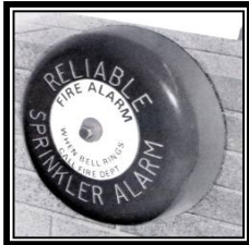
C — Mechanical Spk. Alarm
